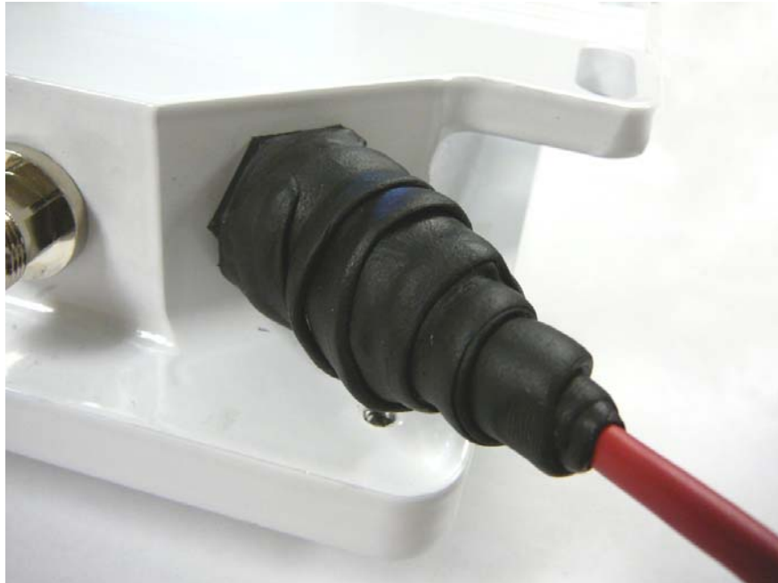
Figure 1: Properly Taped Ethernet Connection
